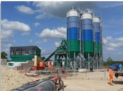
Above; example of batching plant silos
